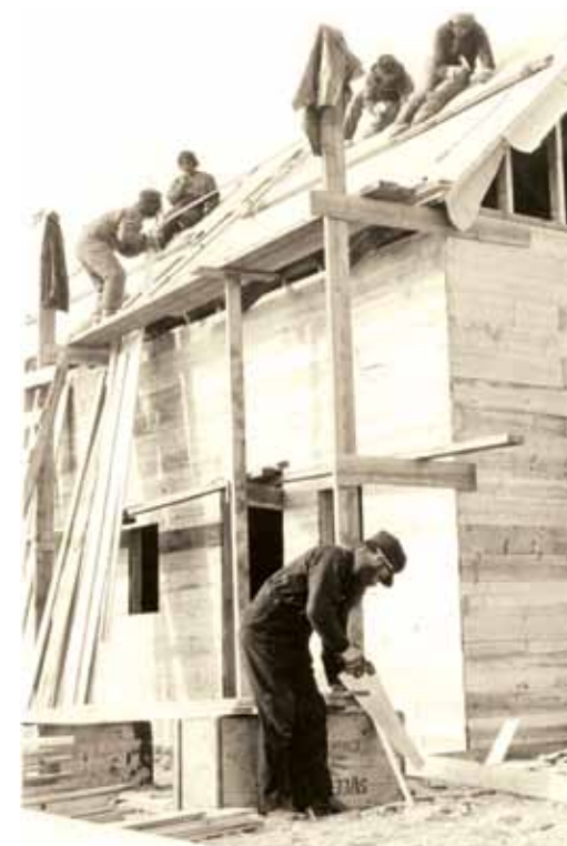
ABOVE Construction of the Roman Catholic Mission Church, Chesterfield Inlet, 1912 - Diocese of Churchill-Hudson Bay CHB 04 0005
